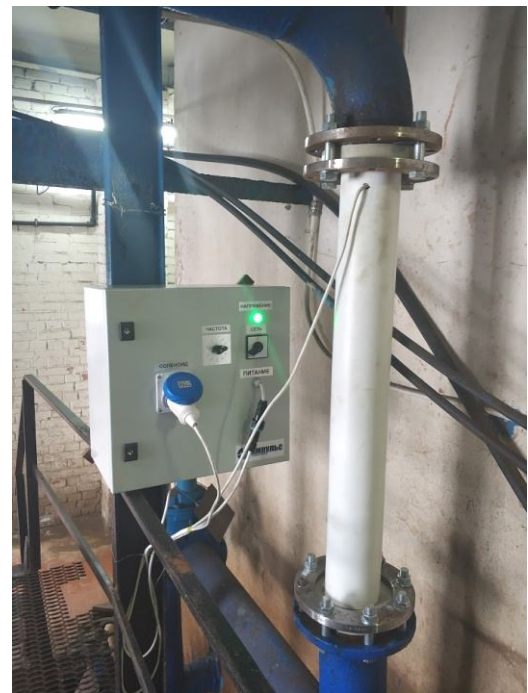
Fig.1. Installation “PMD-2” at the test object
